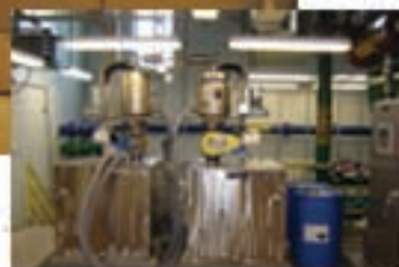
The plant in Lakeville, Minn., came online in March 1998.
